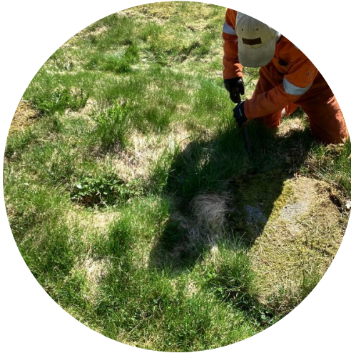
To slamavskillere i betong - sandfilter
